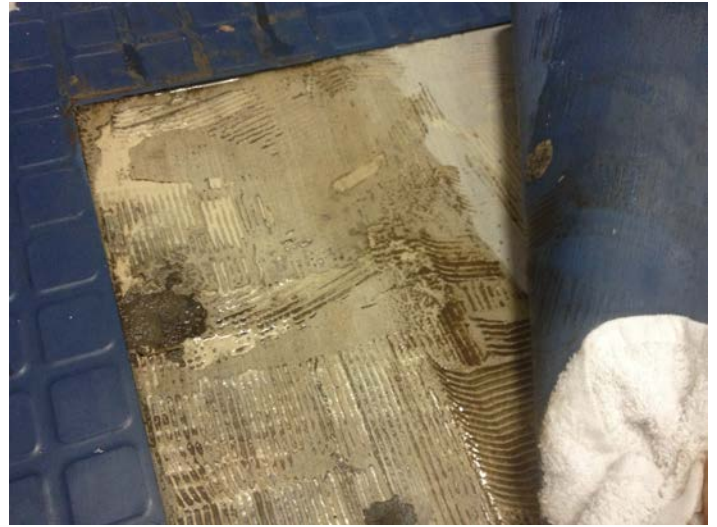
Adhesive loses bond because of moisture & food grease
