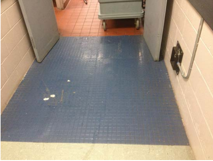
Before, delaminating rubber mats over saturated concrete
