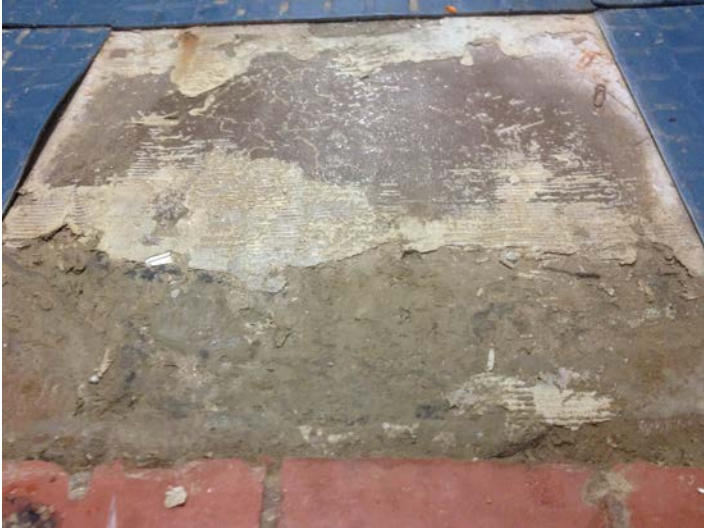
Multiple overlays & improper surface preparation
