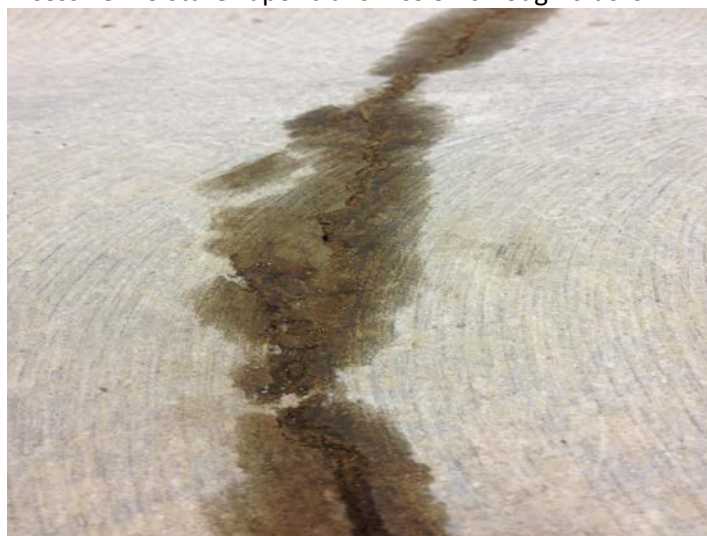
Excessive moisture vapor transmission through cracks
