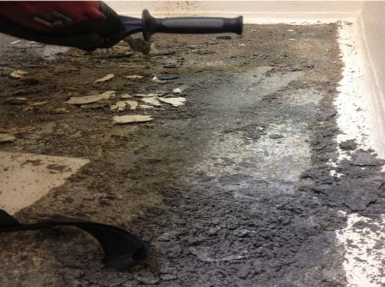
Plumbing fixtures leaks & saturation made for additional challenges
