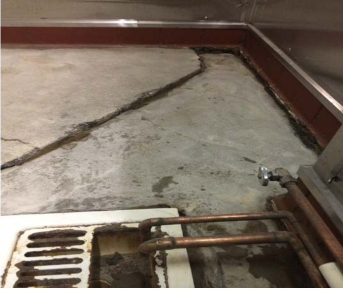
Heavily damage areas pre patched with polymer concrete
