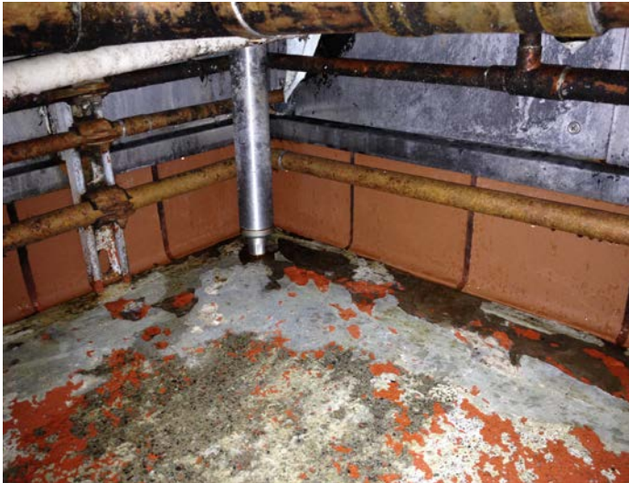
Grease and fats are coming off already
